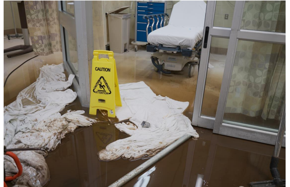
Plumbing system issues resulted in raw sewage in patient care space.
